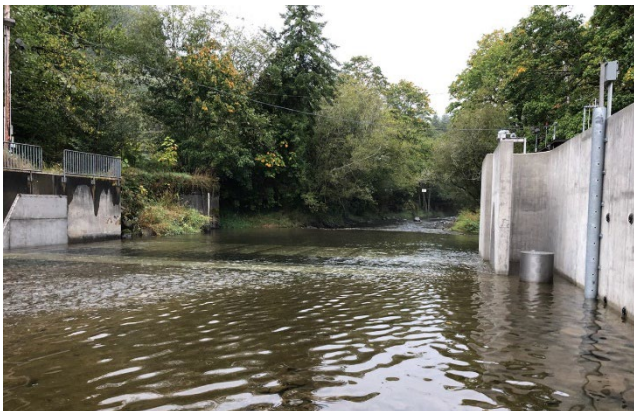
The new adjustable weir lays flat when not needed for hatchery management actions.
